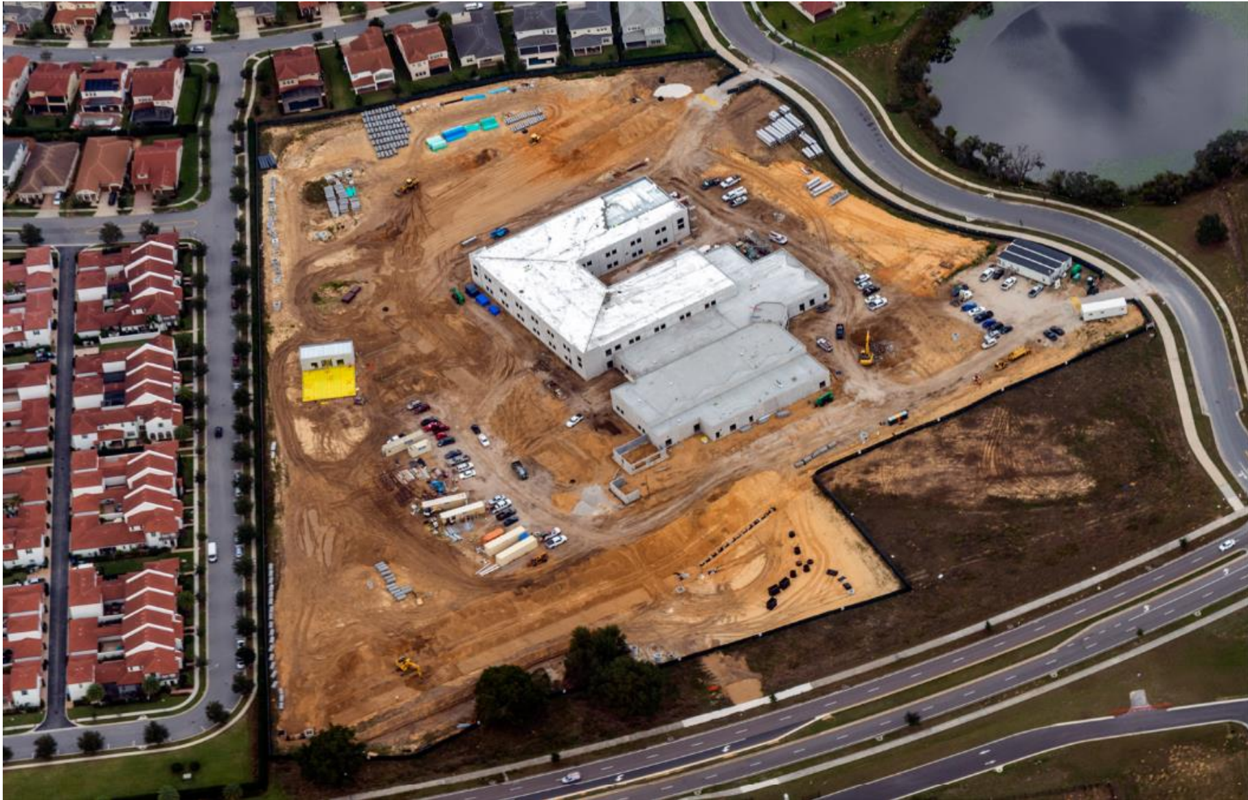
December 2021 – Site 114-E-W-4 : Civil Underground Material Delivery, Metal Decking and Pour LWIC Roofing
