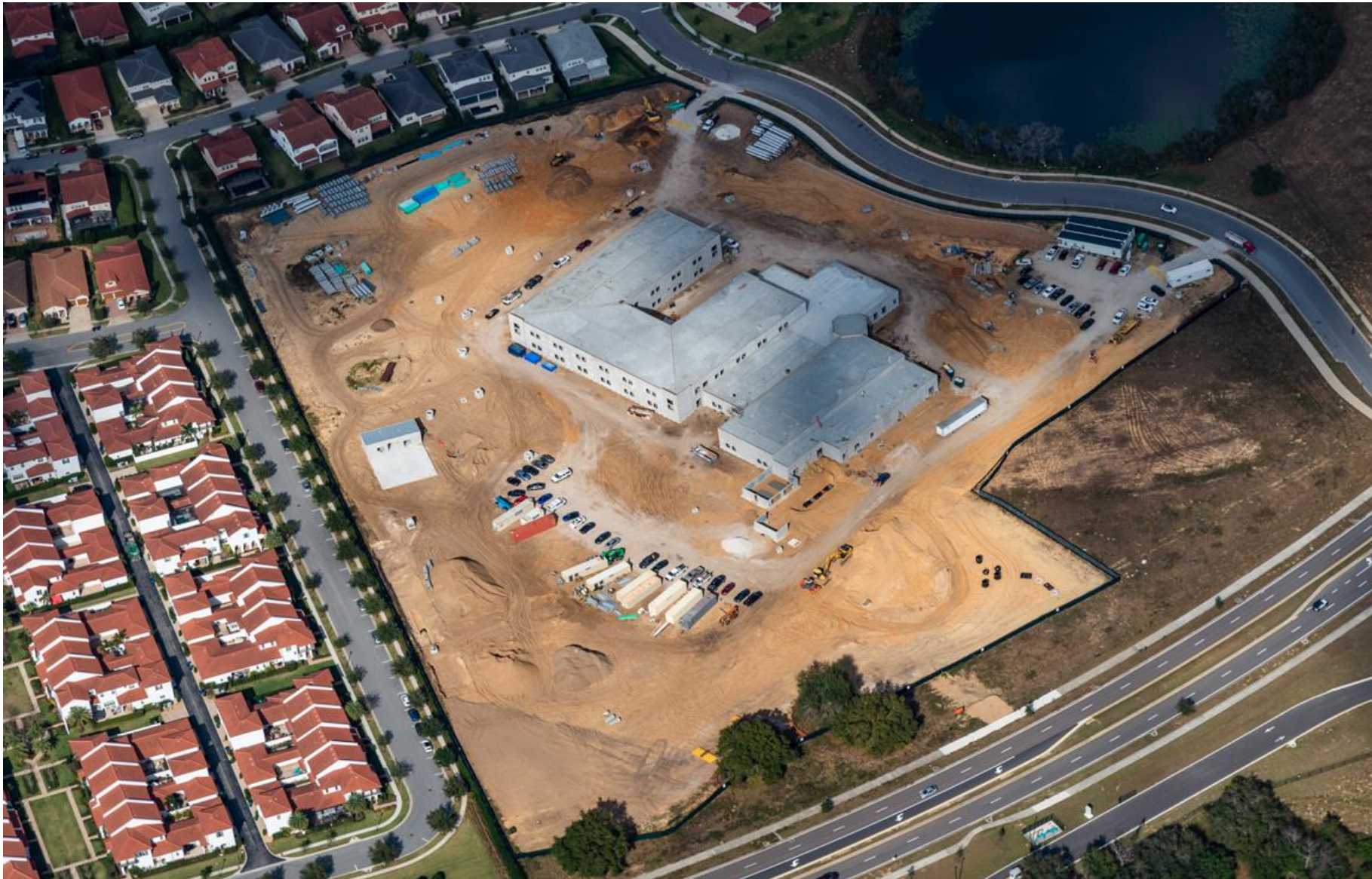
January 2022 – Site 114-E-W-4 : Install Interior Framing and Overhead MEPS. Civil Underground has Started
