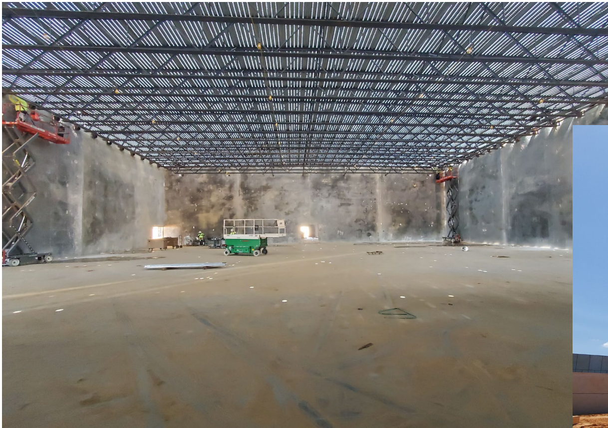
Above is detailing of steel joist and metal decking installation in the Gym
