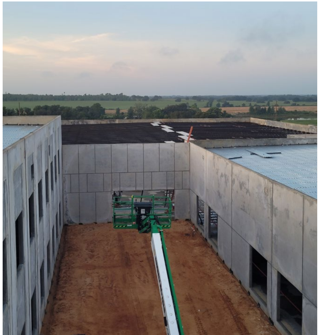
Above is placement of steel joists and metal roof decking of Buildings 5, 1 and 4 from North looking South
