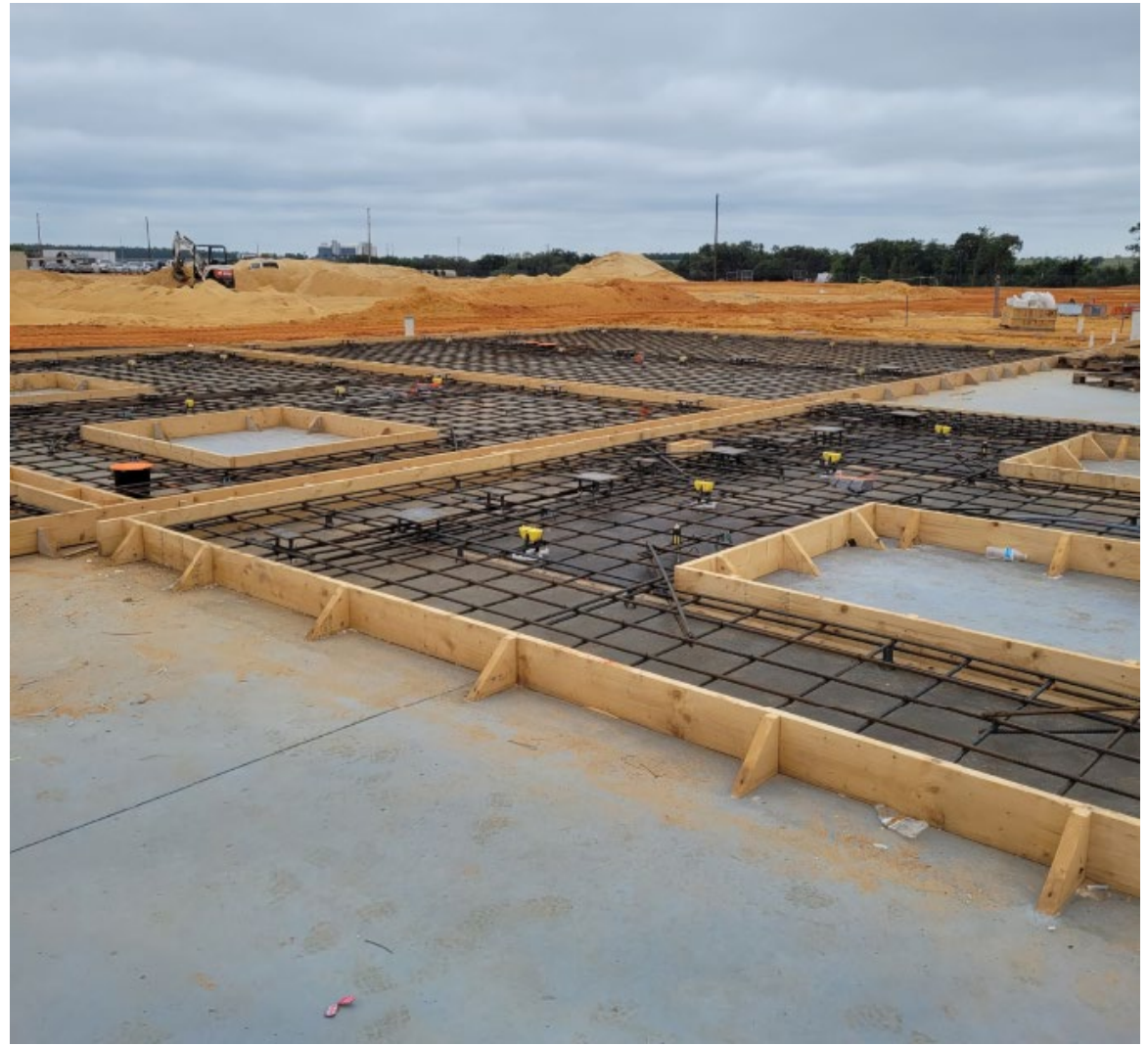
Above is tilt panel formwork with rebar, steel embed and blockout placements
