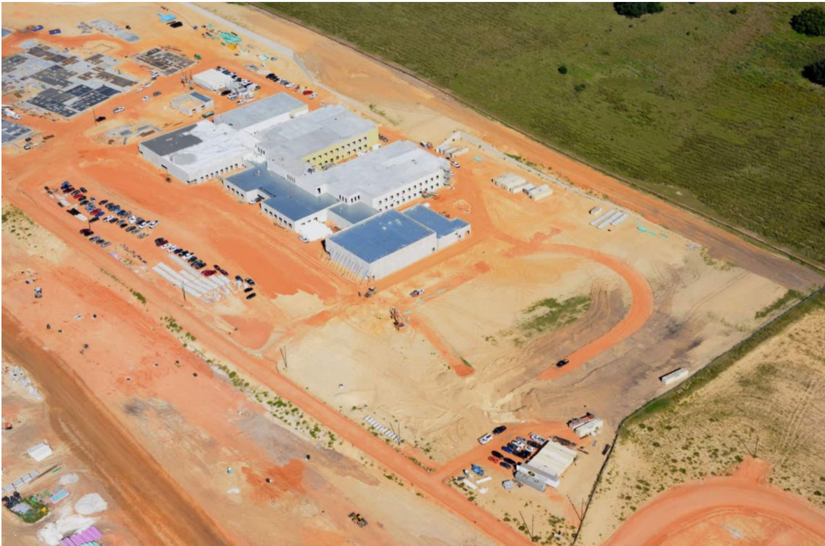
Above is an aerial view from the SE corner looking NW at Site 132 roof prep and prime paint of exterior, and Site 89 tilt panel prep September 2021
