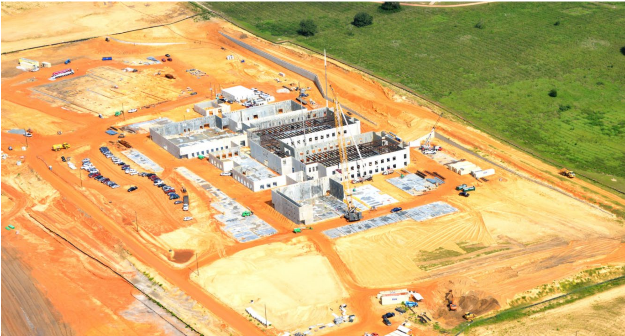
Above is an aerial view from the SE corner looking NW at Site 132 tilt panel erection and steel placement, and Site 89 building foundation prep July 2021
