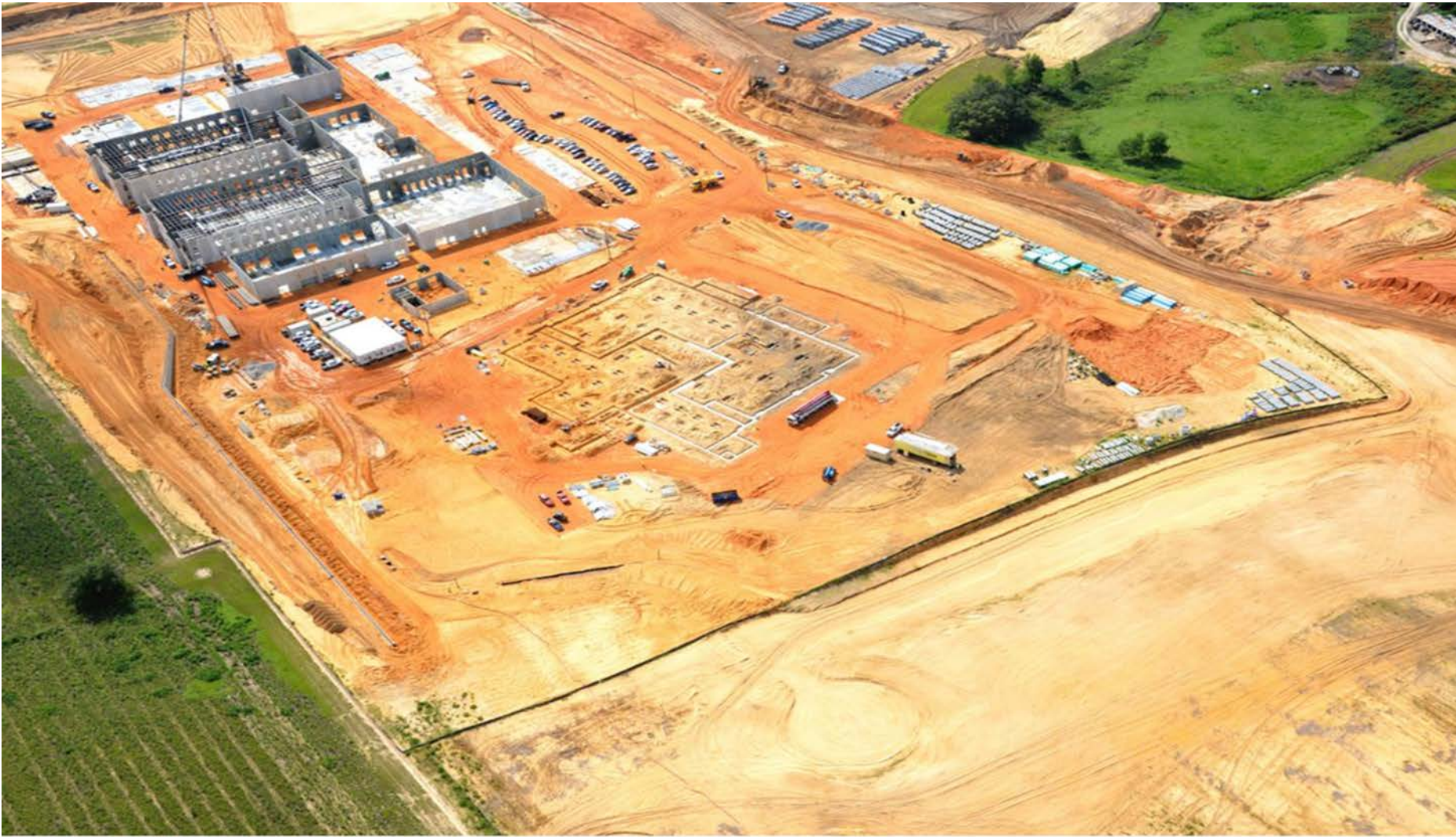
July 2021: Site 89 underground foundations; Site 132 tilt panel erection and steel placement ( aerial view from the West looking East ).
