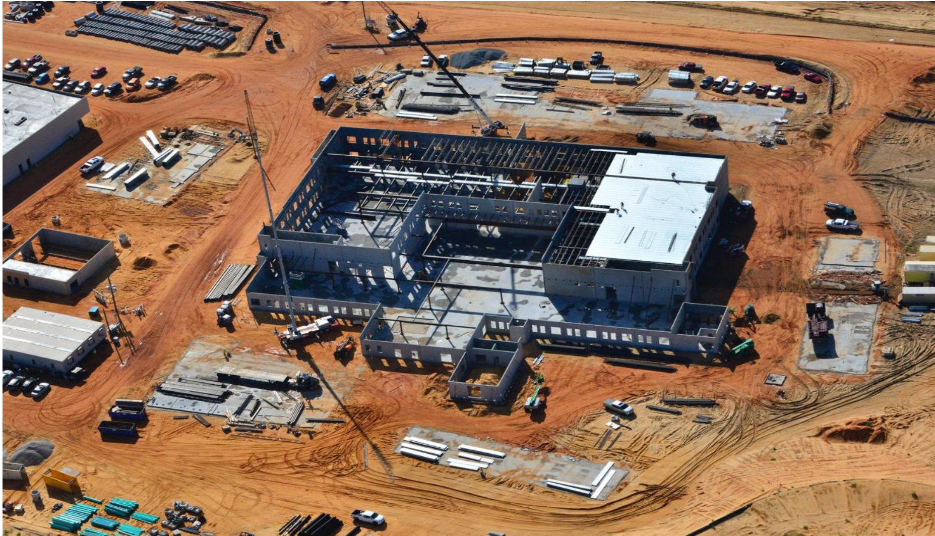
October 2021: Site 89 tilt panels are erected in place and structural steel erection is progress ( aerial view from the Southeast looking Northwest ).
