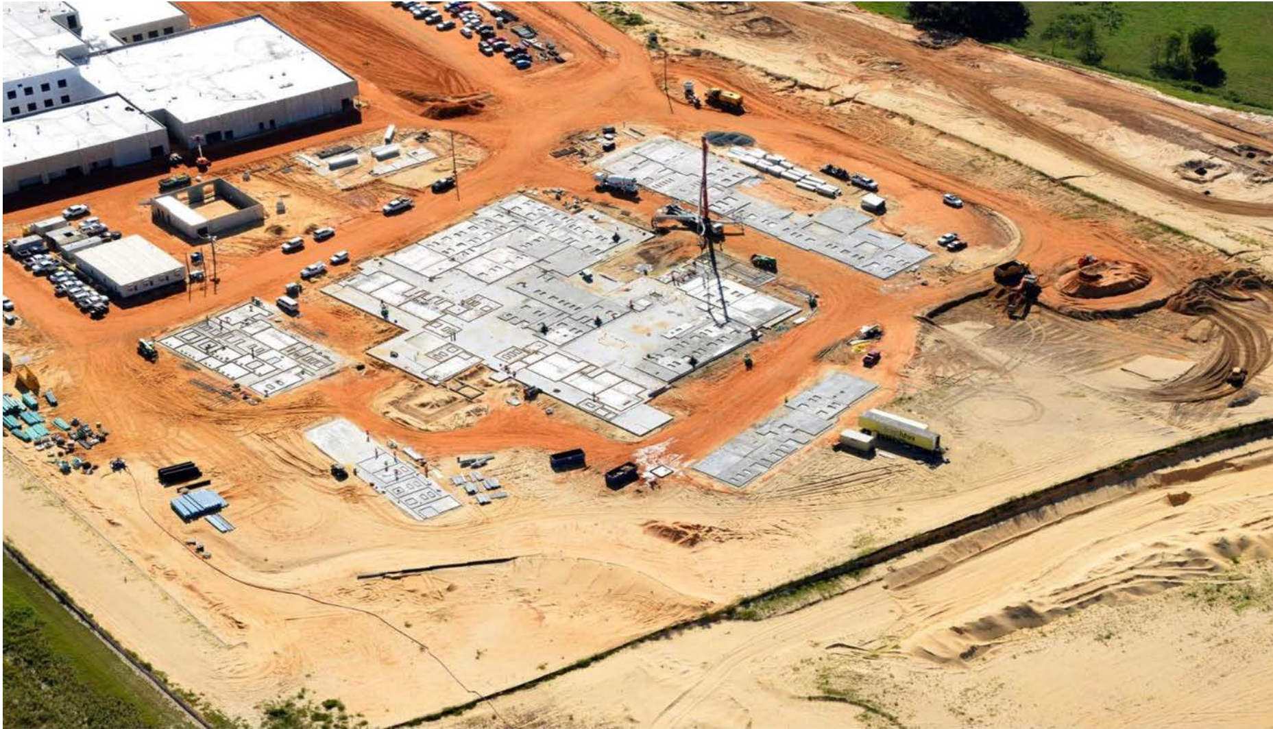
September 2021: Site 89 SOG is poured and the tilt panels are being formed and poured on the SOG/casting beds (aerial view from the Northwest looking Southeast).
