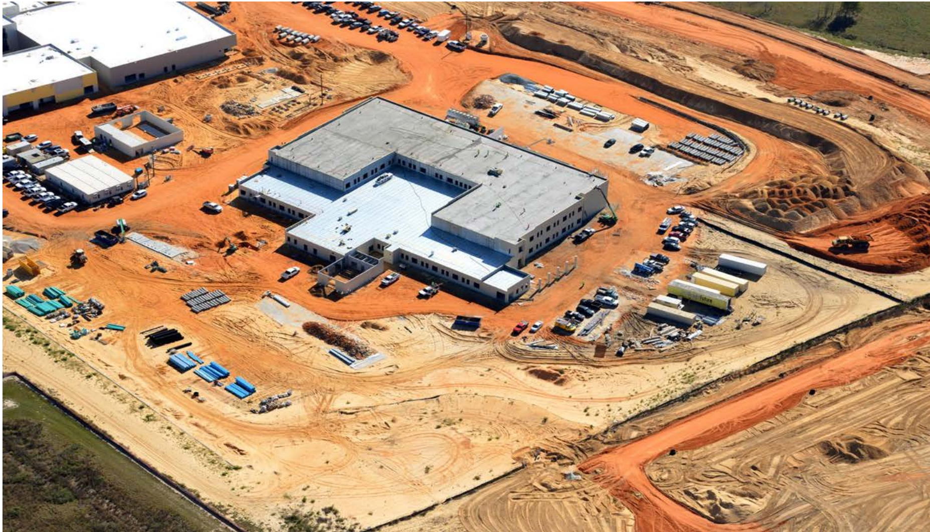
December 2021: Site 89 lightweight insulating concrete (LWIC) installed on High Roof and prepping for install on Low Roof; Covered Play Area columns installed ( aerial view from the Northwest looking Southeast ).
