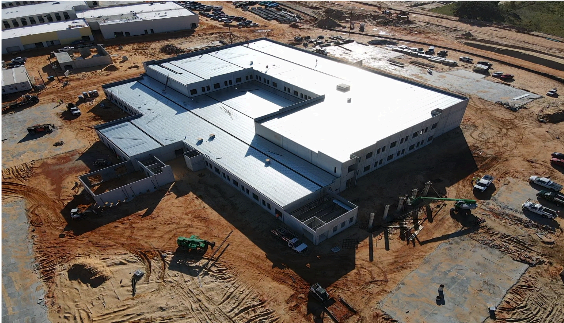
November 2021: Site 89 structural steel install is complete and roof deck is installed ( aerial view from the Southeast looking Northwest ).
