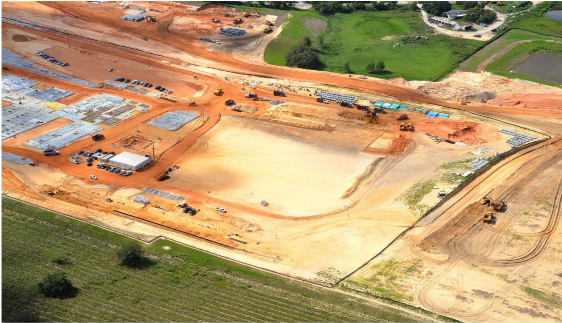
June 2021: Site 89 building pad prep; Site 132 tilt panels on Slab on Grade and casting beds ( aerial view from the North looking South ).
