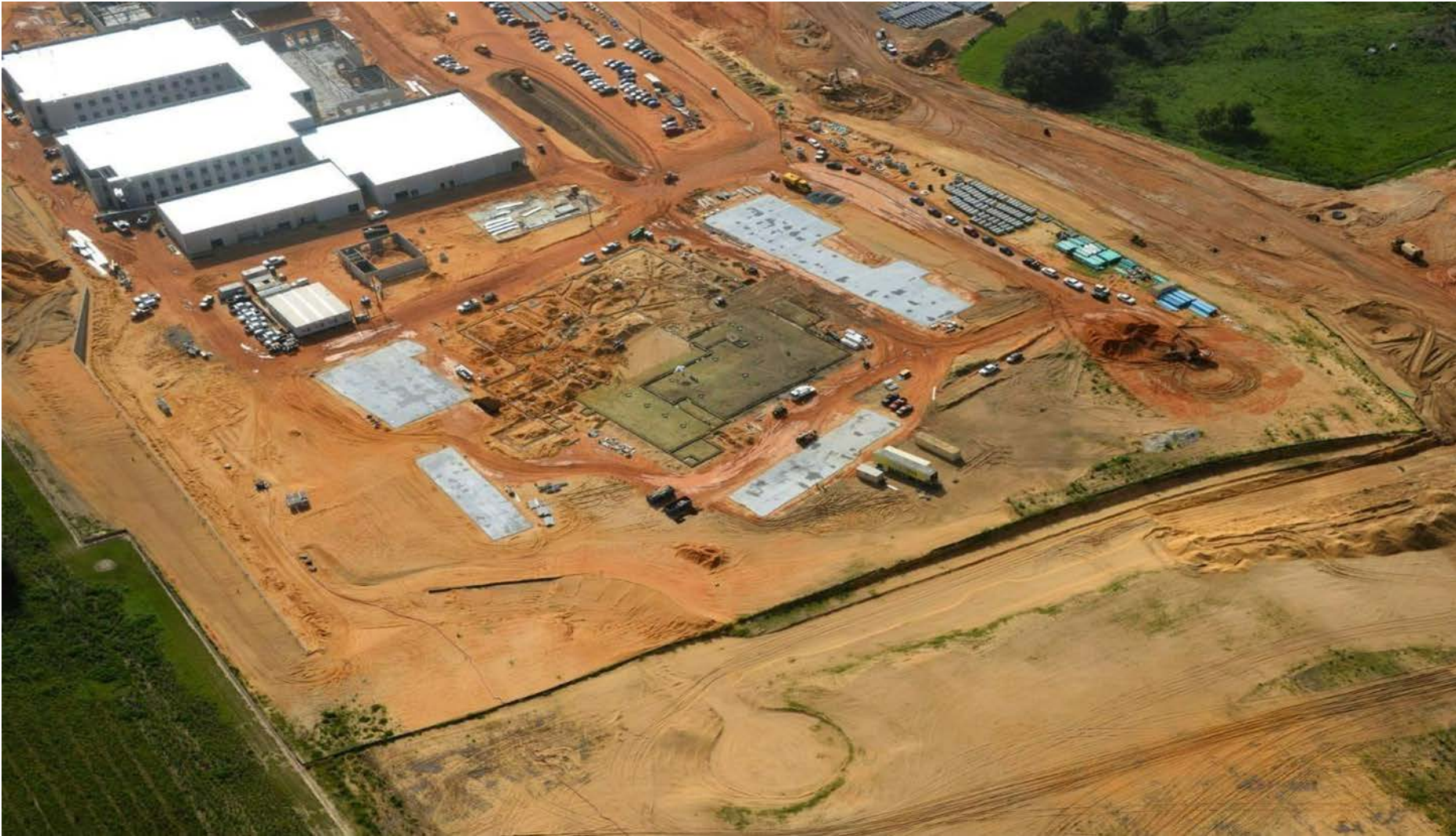
August 2021: Site 89 underground MEP install in progress and prepping for the Slab on Grade Pour #1 ( aerial view from the West looking East ).
